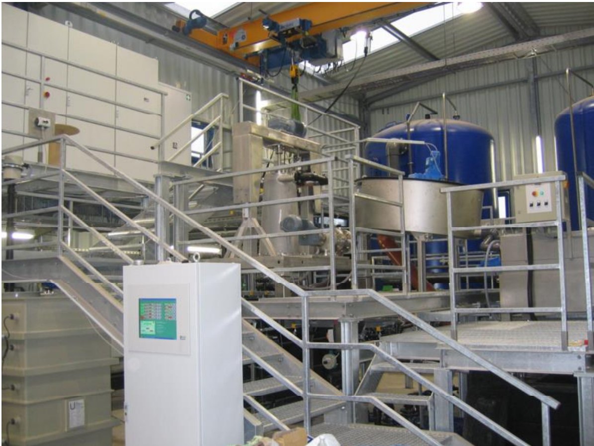
Fig. 12 Partial view of the DeSiFloc system in Hattorf
