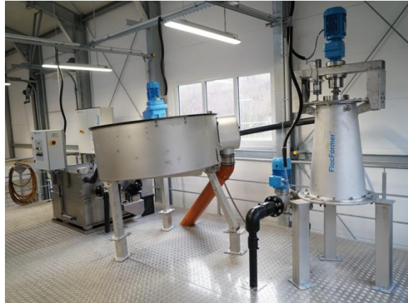
Fig. 13 One line of the DeSiFloc plant in Deiderode
