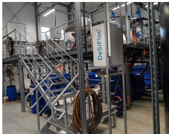
Fig. 14 Partial view of the DeSiFloc system
